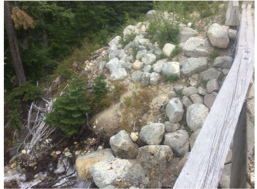
Downstream right bank lack of riprap
