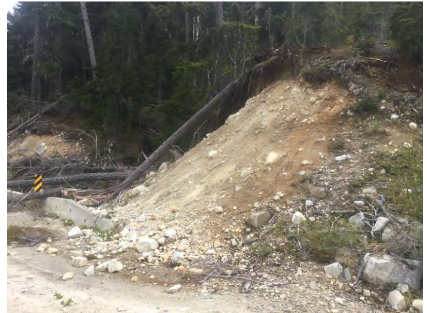
Ravelling cutslope upstream left approach
